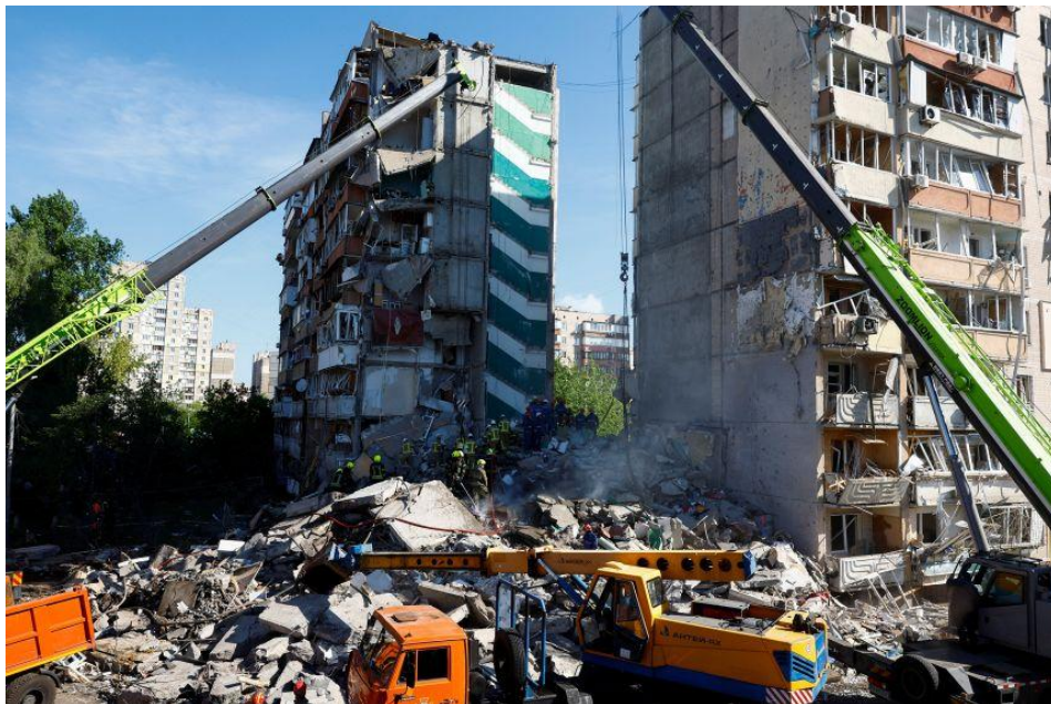
Aerial video shows the aftermath of a Russian attack on an apartment building in Kyiv on May 17. Source: State Emergency Service of Ukraine.
