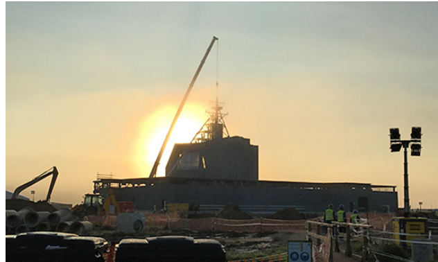
Naval Support Facility Poland – Construction. European Phased Adaptive Approach Phase 3 will enhance the defensive coverage against medium- and intermediate-range threats will be enhanced with the delivery of an Aegis Ashore capability to Poland. The ground-breaking ceremony for Aegis Ashore-Poland was conducted on May 13, 2016. On October 1, 2016, Naval Support Facility (NSF) Redzikowo, Poland was established. (Missile Defense Agency photo)
